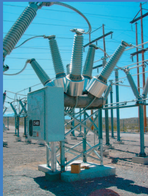
145kV Gas Circuit Breaker
