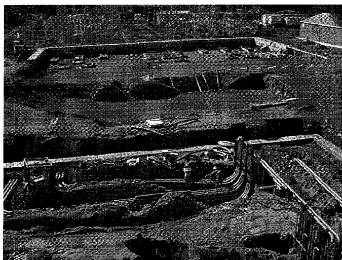
Figure 6. View towards FACTS yard of STATCOM building foundation and conduit work, Essex 115 kV ring bus, and VELCO building (upper right) (July 2000).
