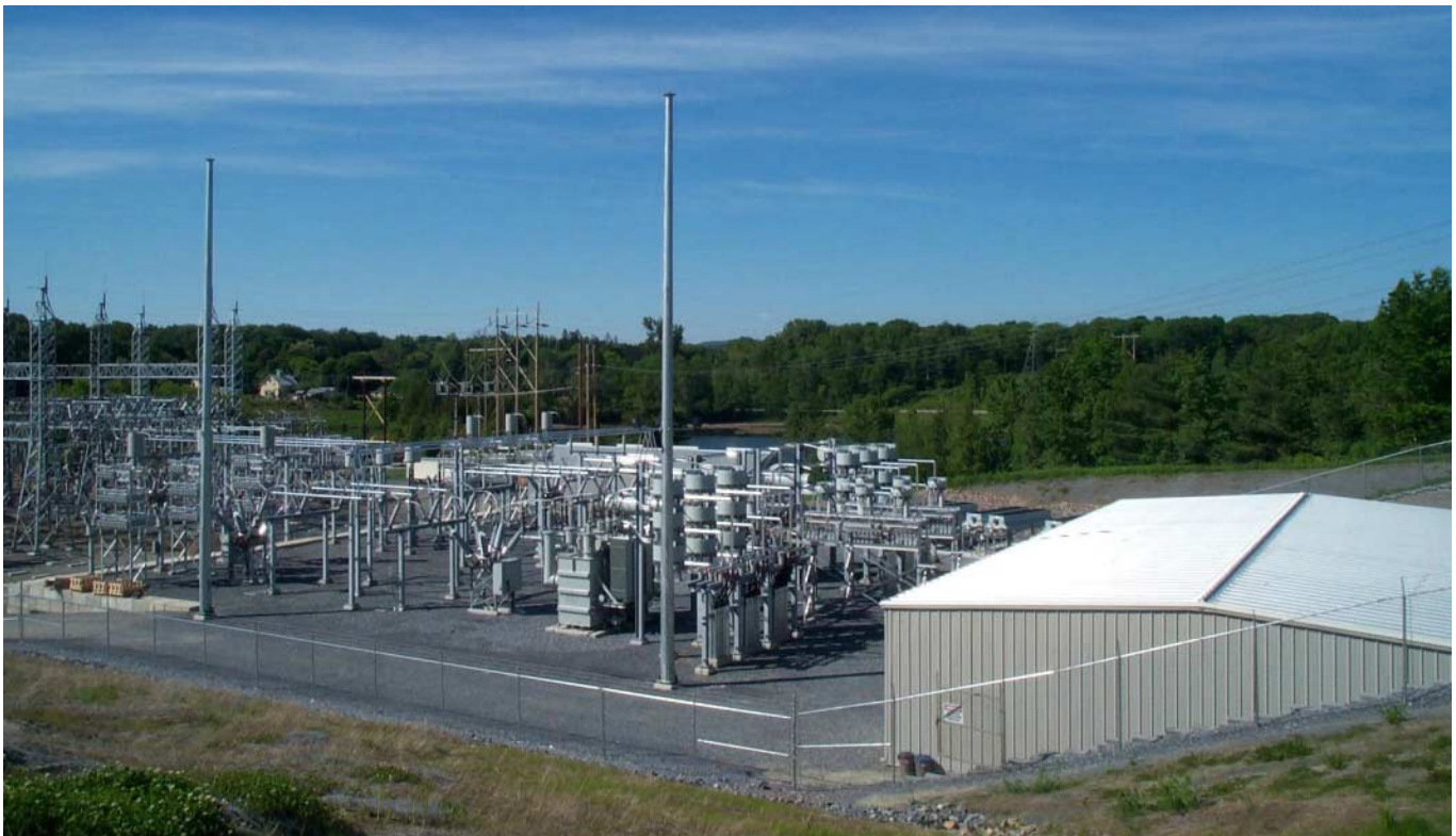
Figure 1. VELCO Essex +133/-41 MVA, 115 kV STATCOM system
