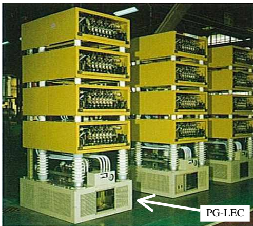
Fig. 5. The thyristor valve photograph of Shin-Shinano SVC
