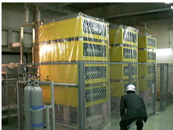
Fig. 6. The thyristor valve photograph of Suruga SVC
