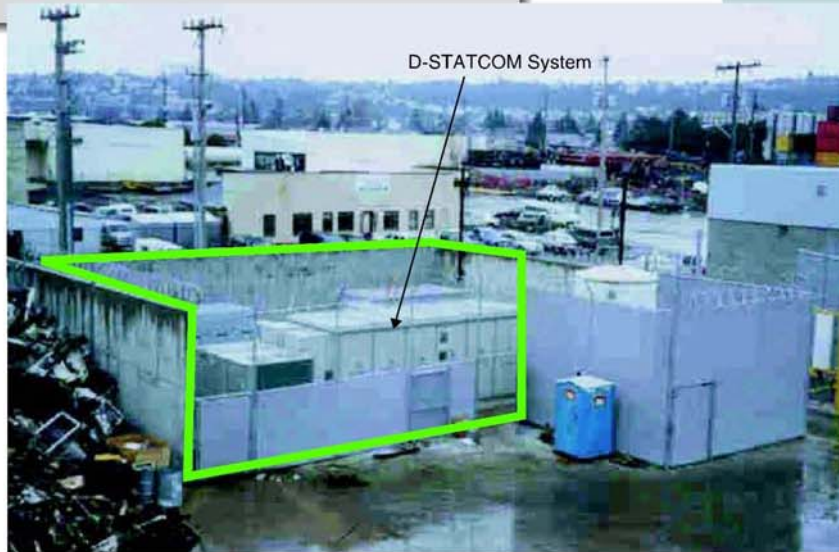
Seattle Iron & Metals D-STATCOM -External View at Steel Recycle Facility
