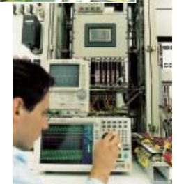
Site Tests Performance tests are carried out combining all controllers and protection devices and all AC and DC auxiliary equipment.
