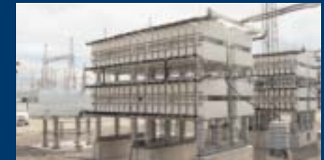
6 Capacitor Bank 7 Filter Reactor
